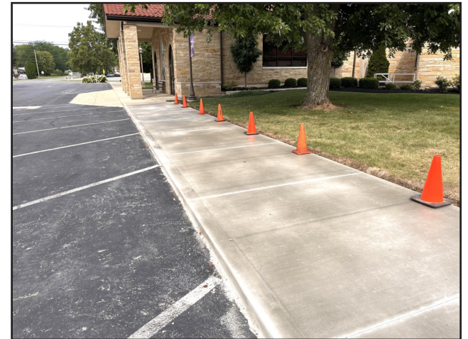
A much-needed new sidewalk is being installed along the Southeast corner of the church, ensuring a safer path for our parishioners.
